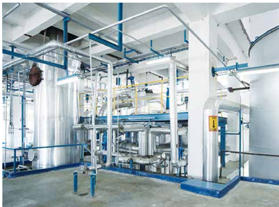
Integrating the upstream melt production process gives the manmade fiber manufacturer optimal influence on the entire production chain.
