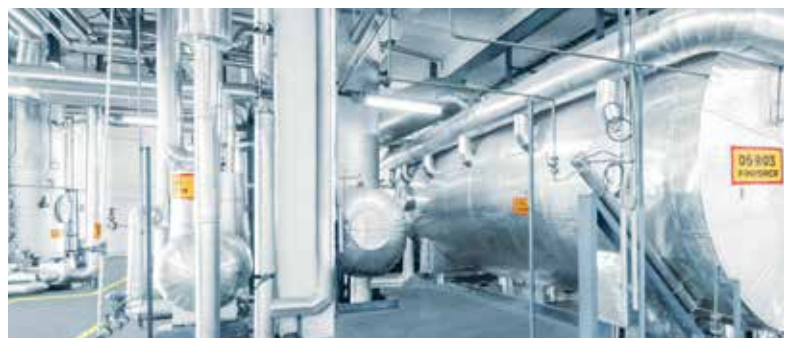
The industrial yarn project at Jiangsu Solead has become a 'From Melt to Yarn' total solution with the commissioning of the polycondensation system.
